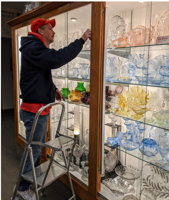
The new vertical LED case lights look wonderful. Ben Kirkman has done a great job with the installation and ballast removal.
