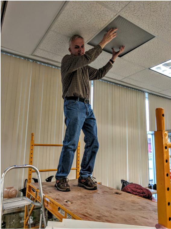
Greg Vass climbed up on the scaffolding to remove the ceiling vent for cleaning.
